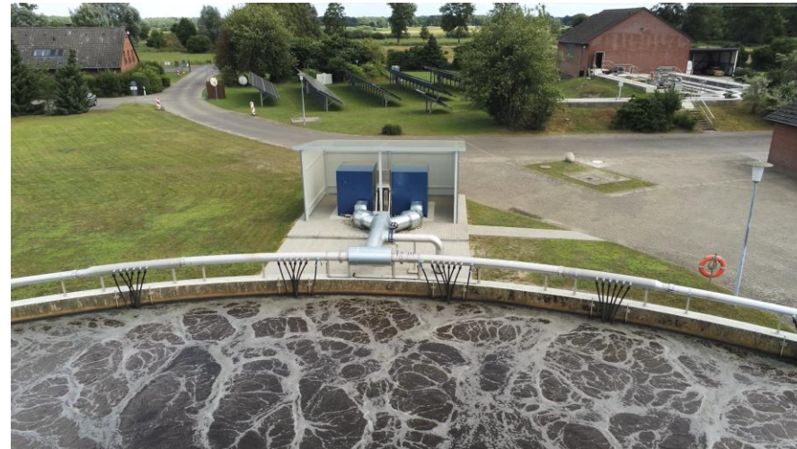
Aeration basin and Aerzen compressor system of WWTP Liebenwalde
